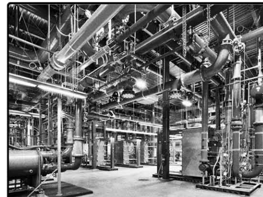
Facebook Data Center at Prineville, Oregon (above) image source: http://www.highsnobiety.com/2012/10/25/a-look-inside-the-facebook-data-center/
