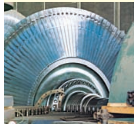
Thermal power station at La Casella
