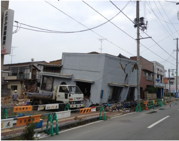
Earthquake damage in Minamisoma
