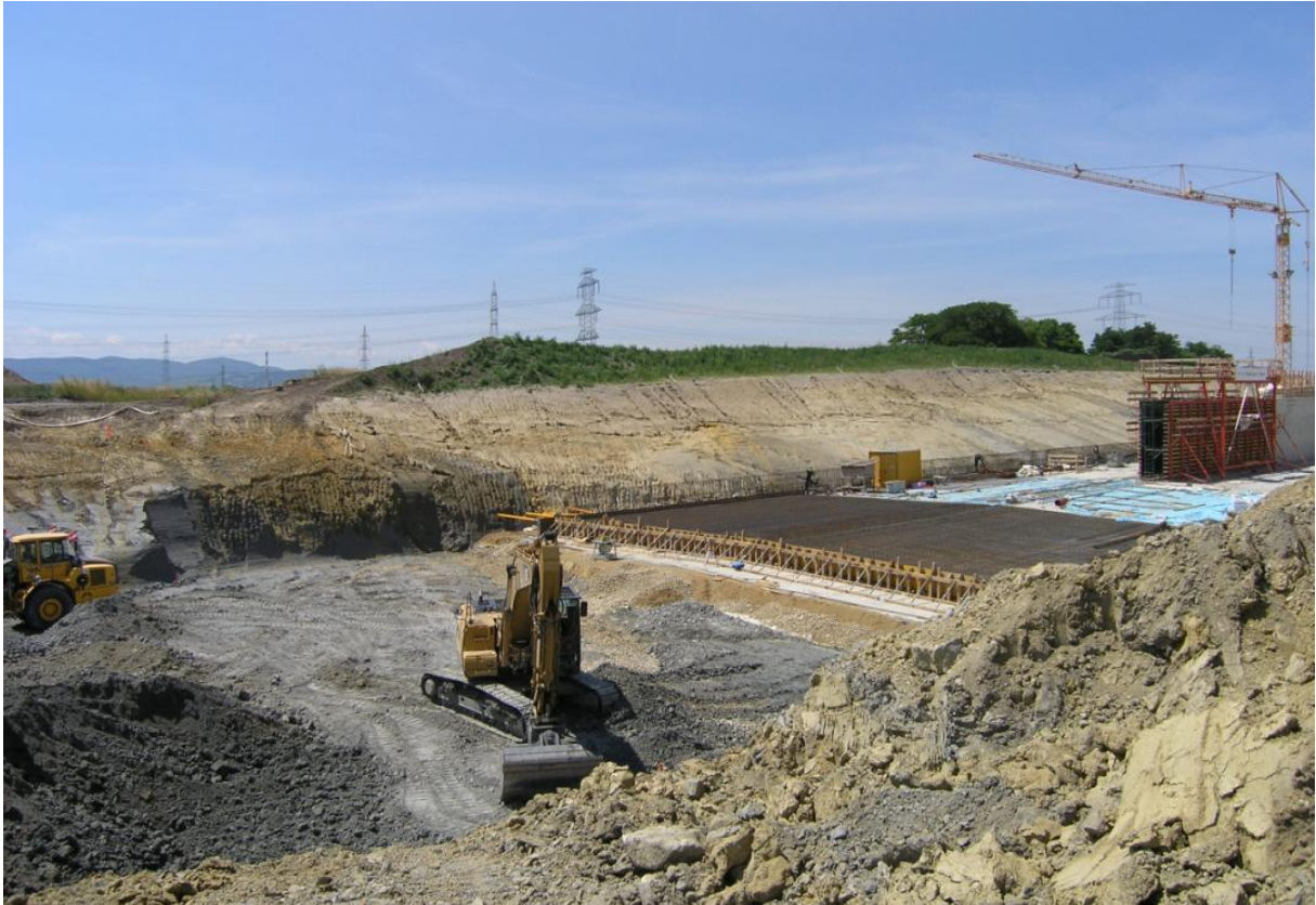
Figure 8: Sampling was conducted along the road construction site of the S1 (photography provided by H. GEBHARDT, GBA).
