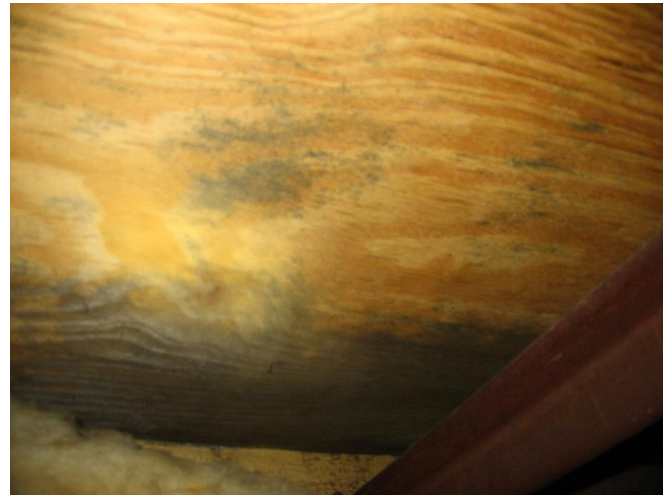
Figure 2 Scattered black spots of mould growth on a section of the plywood sarking
