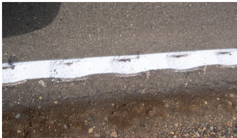
Figure 26. Completed edge-line rumble stripe on a rural highway in Iowa (Hallmark et al. 2010)
