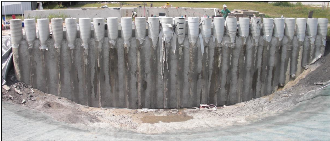
Figure 7.37: Water infiltration into the excavation was first observed 90 minutes from the start of inundation.
