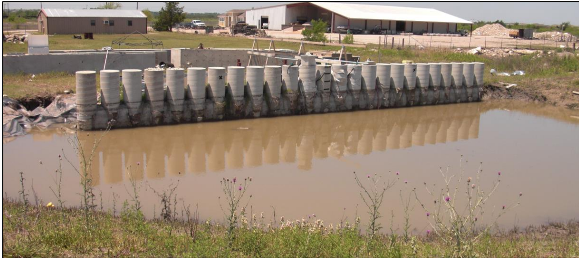
Figure 7.4: Flooding in response to a large storm before the May 6, 2013 data surveys. Water level in the excavation reached ground surface.
