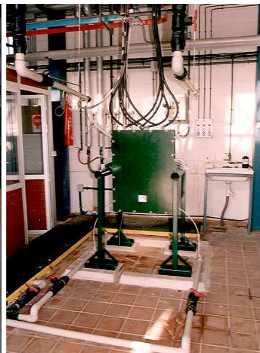
Electrochemical pilot plant, Applied electrochemistry laboratory, University of Alicante
