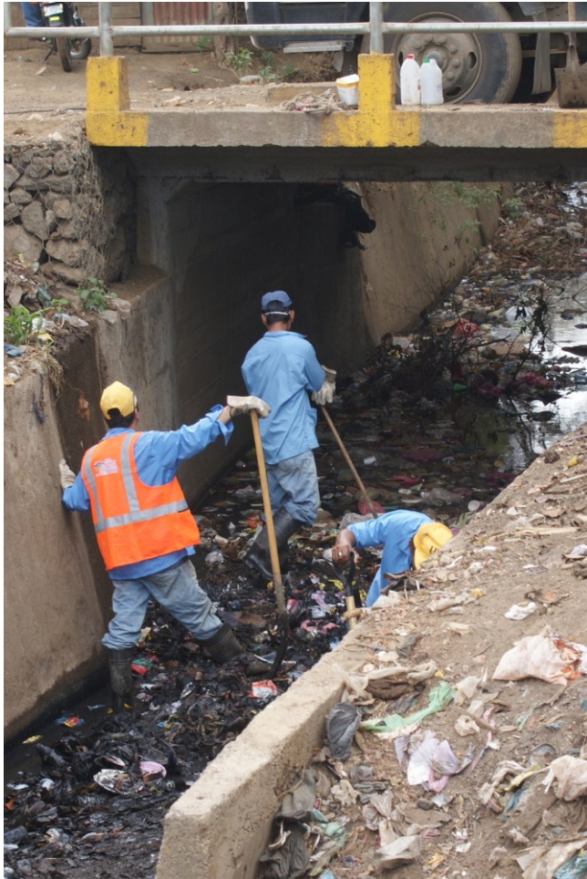
in a storm canal is being cleaned in preparation for the rain season
