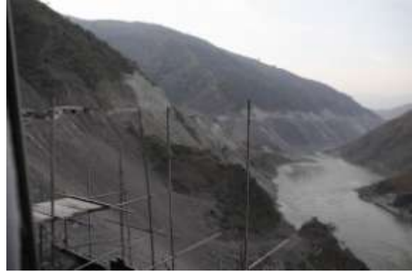
Construction of the Ludila power plant on the Jinsha River (both photos: WangYC 2008)
