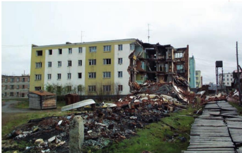
Figure 10. Irregular settling due to permafrost thaw destroyed this apartment building in Cherski, Siberia (photo: Vladimir Romanovsky, in Schaefer et al., 2012).
