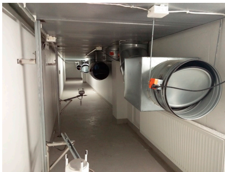
Figure 4. Supply air duct corridor and classroom-specific ducts' terminal units in the basement. Dampers are opened 20%, as designed.
