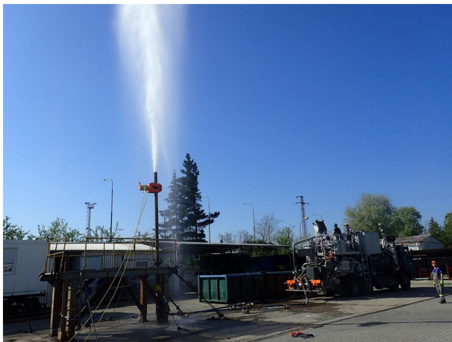
Figure 7. The premises of HBZS Hodonin. The elimination of open eruption by drilling tools with help of apparatus FIB-1 and designed sealing elements.
