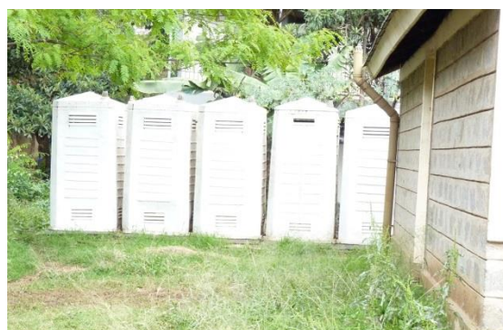
Photo 7.2 Eco-Toilet (R) at Toi Primary School
