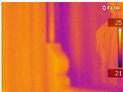
Fig (g): heat leakage around window frame
