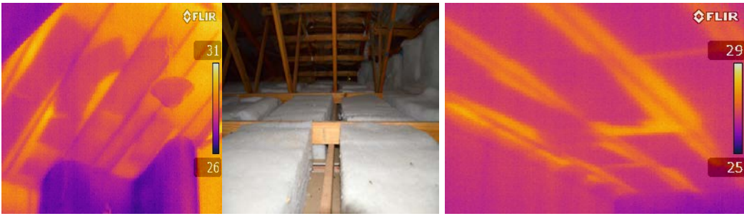
Figure 5.8: Missing insulation as well as large air gaps around insulation, representing serious breaches of BCA regulations
