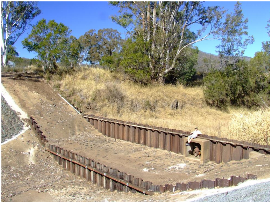
Figure 92. Mulgowie recharging weir in 7/2007. Laidley Creek completely dry along its whole course.
