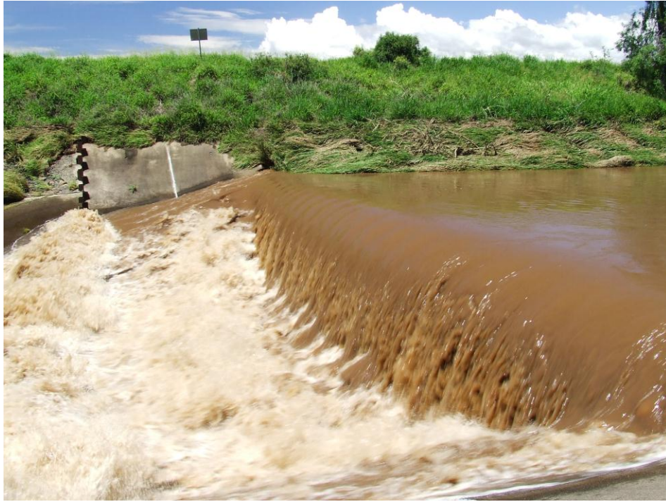
Figure 91. Laidley diversion weir in 11/2008. Flattened grass indicates the maximum height of the flood.
