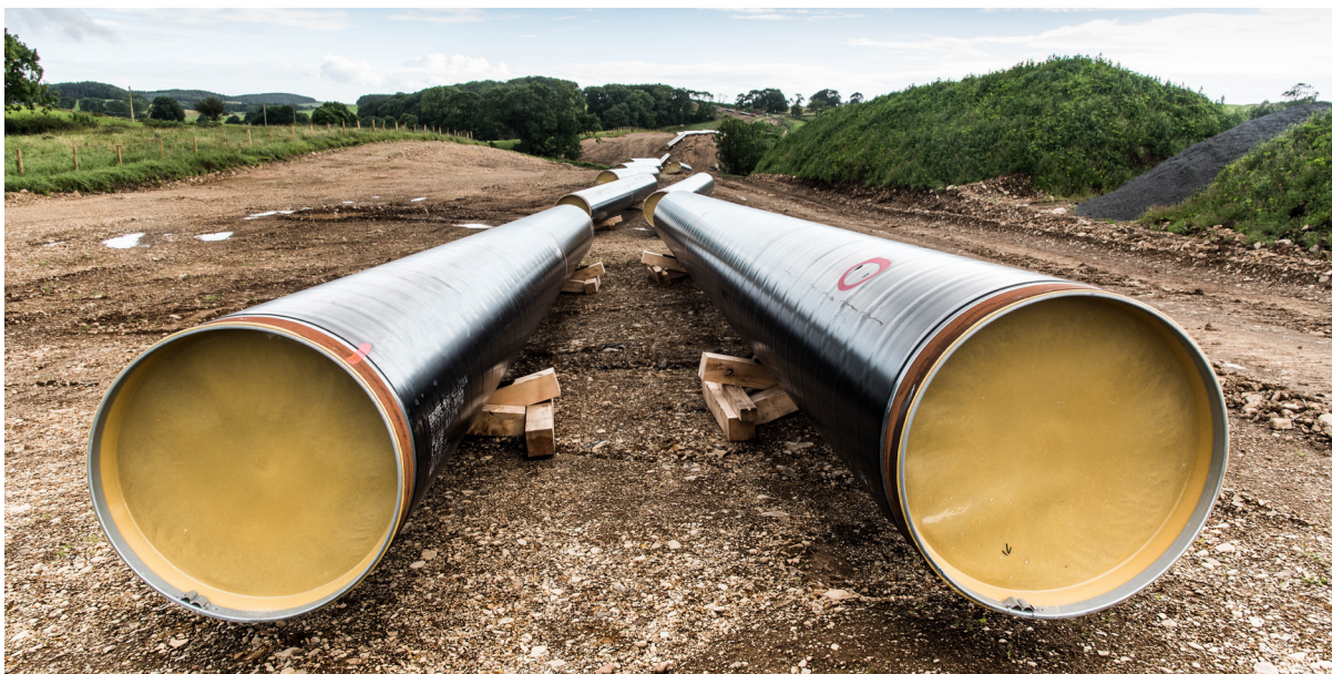
Construction of a pipeline between Cluden and Brighthouse in Scotland, as part of the Scotland-Ireland interconnector project that has recently received financing from the European Investment Bank
