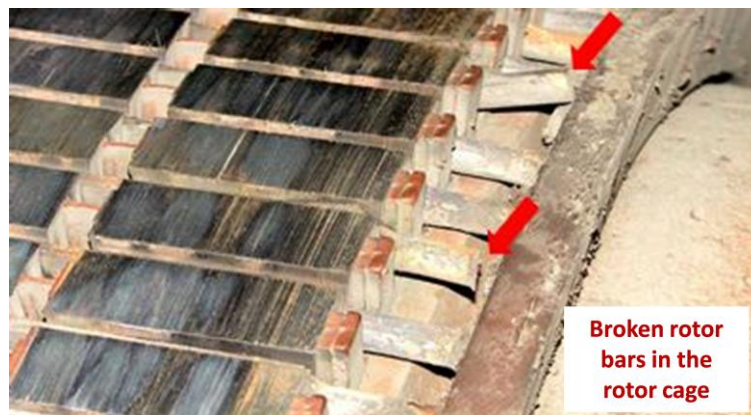
Fig. 1. Evidence of two broken bars in the rotor of an induction motor
