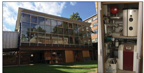
Figure 1. Photos showing the Architecture Studio building (left) and the energy supply system cabinet with the heat pump on the bottom and the buffer tank on the top.
