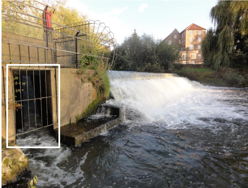
Figure 2.3. Stamford Bridge weir. The white outline indicates the location of the Denil fishway entrance. Photograph taken on 07/10/2011.
