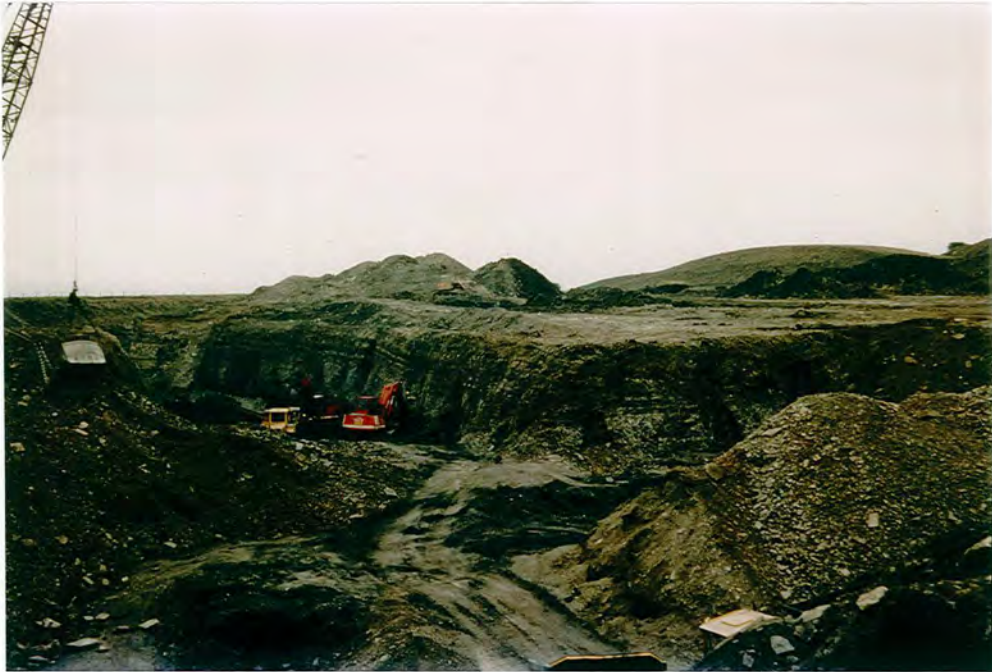
Plate I.5 - View showing excavation of solid rock, and dumping of rubble in earlier "cuts" - Mown Meadows O.C.C.S.
