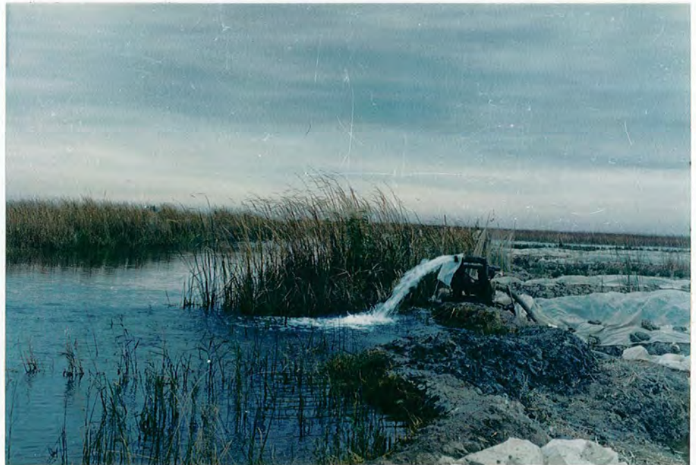
FIGURE 5.15 : Pumping of excess water from the main ditch into the main canal
