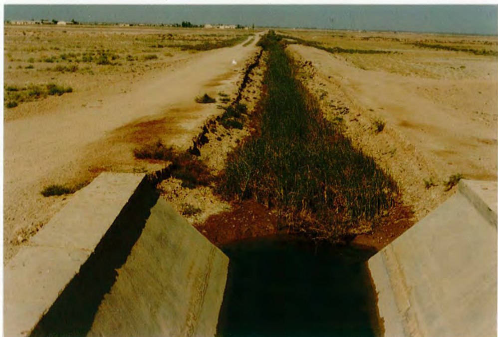
FIGURE 4.16 The weed growth and sediment accumulation in a secondary canal
