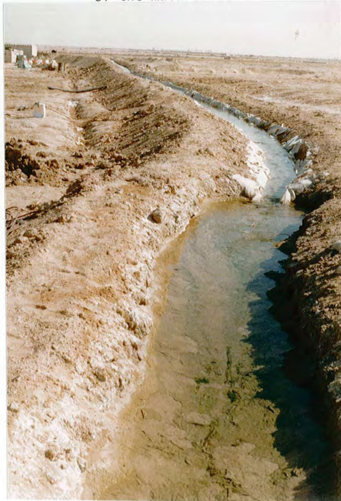
FIGURE 3.7 : Use of plastic sheets to line some portions of the main canal
