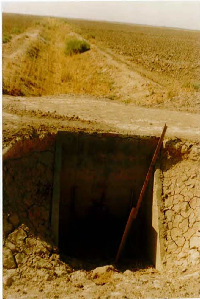
FIGURE 4.17 : One of the neglected joints and canals
