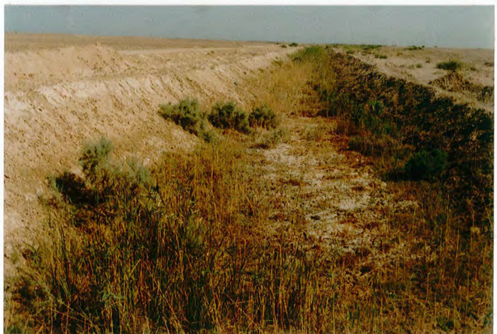
FIGURE 4.18 : One of the neglected secondary drains
