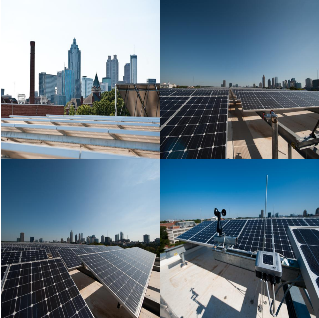
Figure A.1: Pictures of 86.4 kW PV system on Clough Commons.
