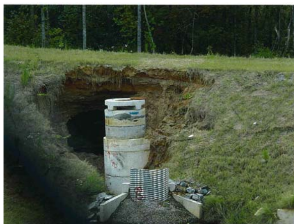
Figure 3. Dam Failure at Outlet Structure
