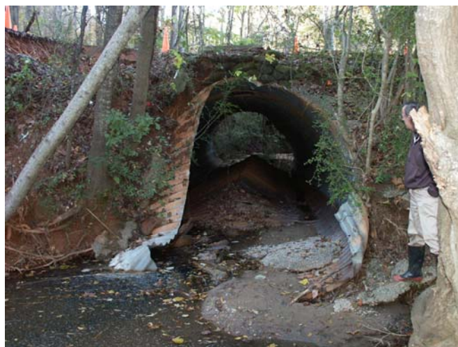
Figure 2: Failing Storm Pipe in Troup County
