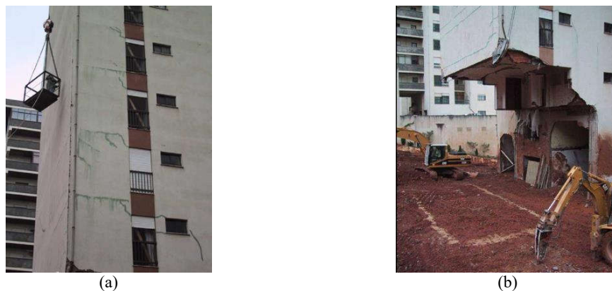
Figure 2 –Details of the accident: (a) cracks along the façade masonry infill walls; (b) removal of debris from the accident site.
