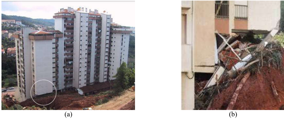
Figure 1 –Severely damaged RC residential building after a land slide: (a) rear façade; (b) collapse of the outer columns of the rear body of building.
