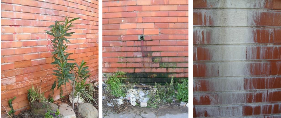
Figure 10. Most common defects in ceramic claddings due to the presence of damp.
