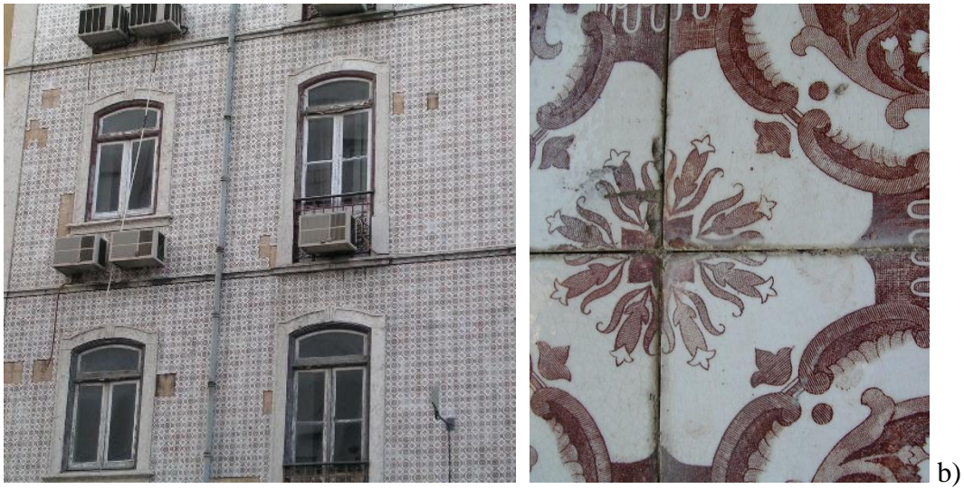
Figure 11. Illustrative example of the influence of the exposure to the wind-rain action in the degradation condition of ceramic claddings.
