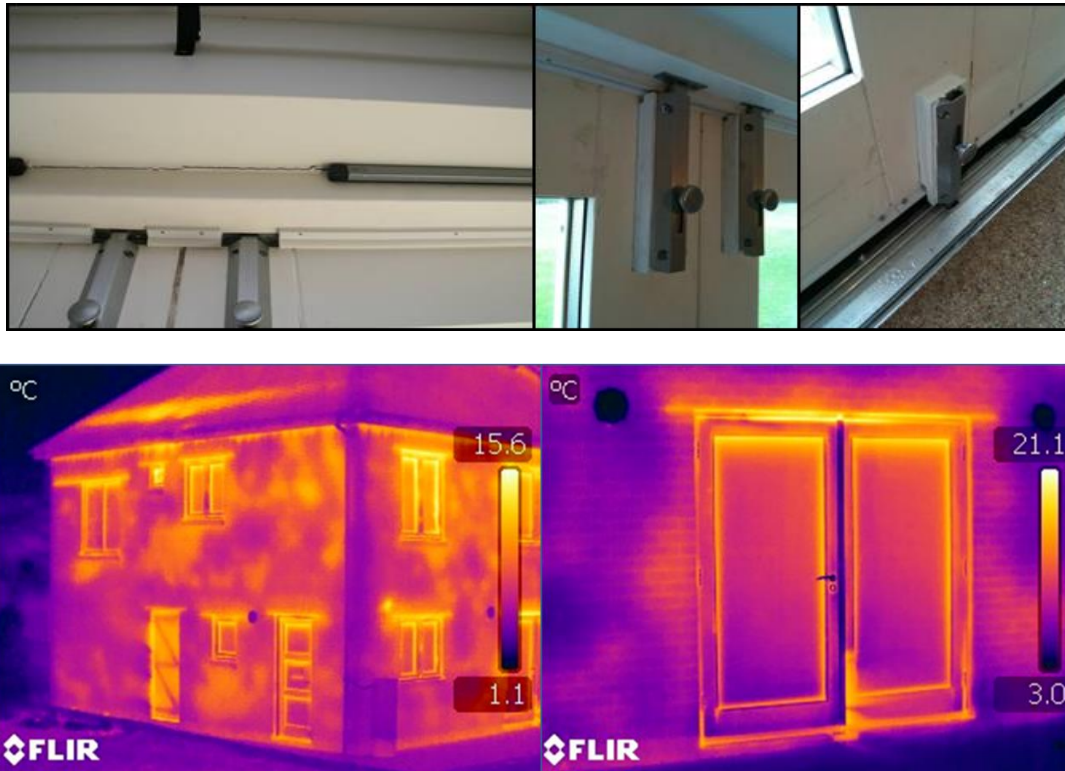
Figure 6 – Observational evidence of poor quality installation and of uneven cavity wall insulation.
