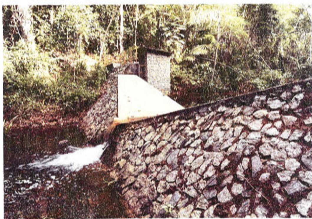
c) Detailed view of the weir in MBE area used in the runoff measurements
