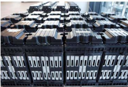
Figure 6: Li-Ion battery energy storage system installed at EKZ Dietikon, Switzerland [4]
