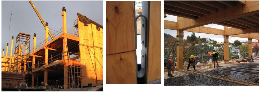
Figure 20. World First Pres-Lam Building. Nelson Marlborough Institute of Technology, (NMIT), Nelson, New Zealand. Post-tensioned timber (Pres-Lam) walls coupled with U-shape Flexural Plates (UFPs) (Structural Engineers Aurecon; Architects Irving-Smith-Jack, Devereux et al., 2011)
