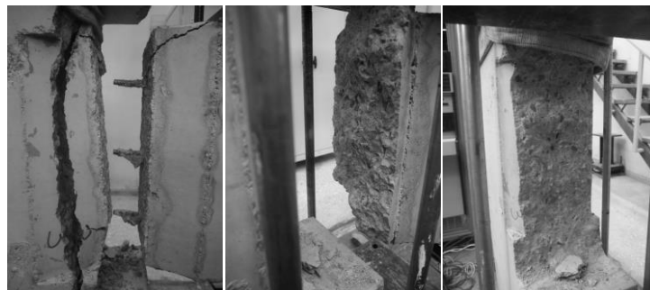
Figure 4. Formation of a second crack, parallel to the interface. The crack occurs close to the back end of the (short) reinforcing bars. Observe the formation of concrete cones.
