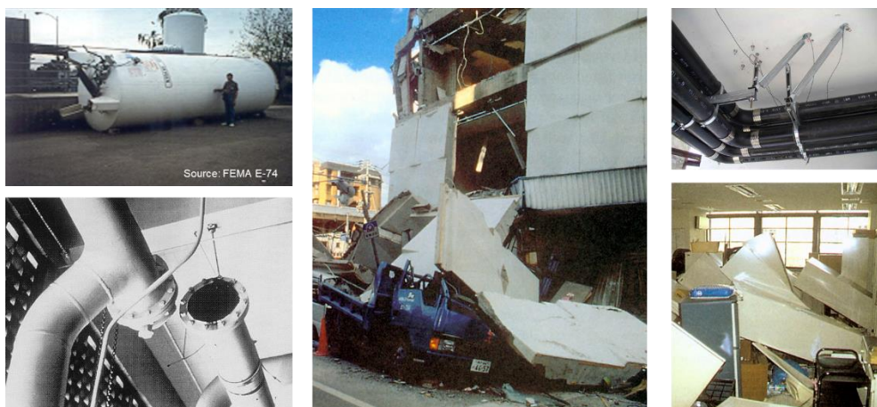
Figure 3. Examples on anchor failures (nonstructural)
