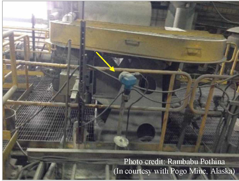
Figure 1.2: A level sensor from Pogo flotation circuit.
