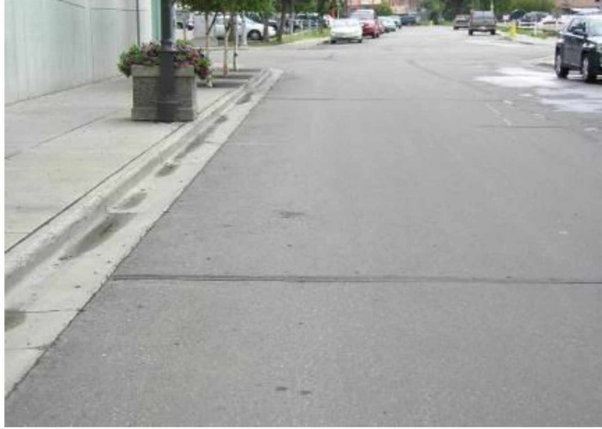
Figure 3.8: 3rd Avenue, Fairbanks, crack seal, thermal cracking, 2011.
