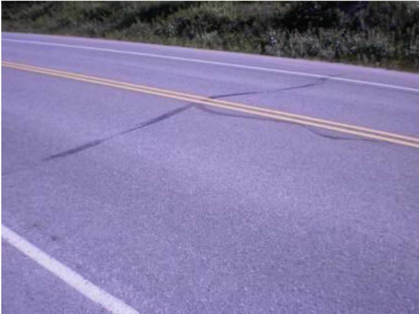
Figure 3.1: Abbott Road, Anchorage, crack seal, thermal crack and frost damage, 2011.
