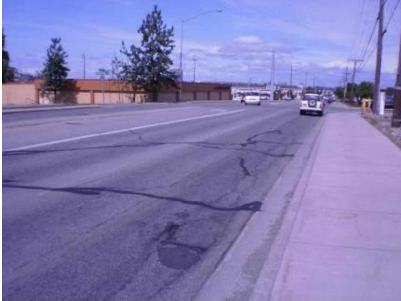
Figure 3.2: Old Seward Highway, Anchorage, crack seal, thermal and frost damage, 2011.
