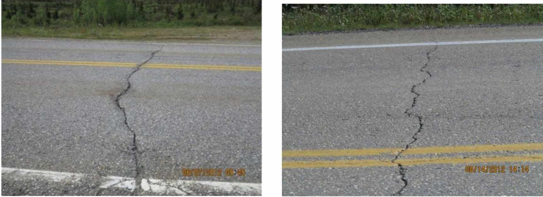
Figure 3.13: Examples of major thermal cracks.
