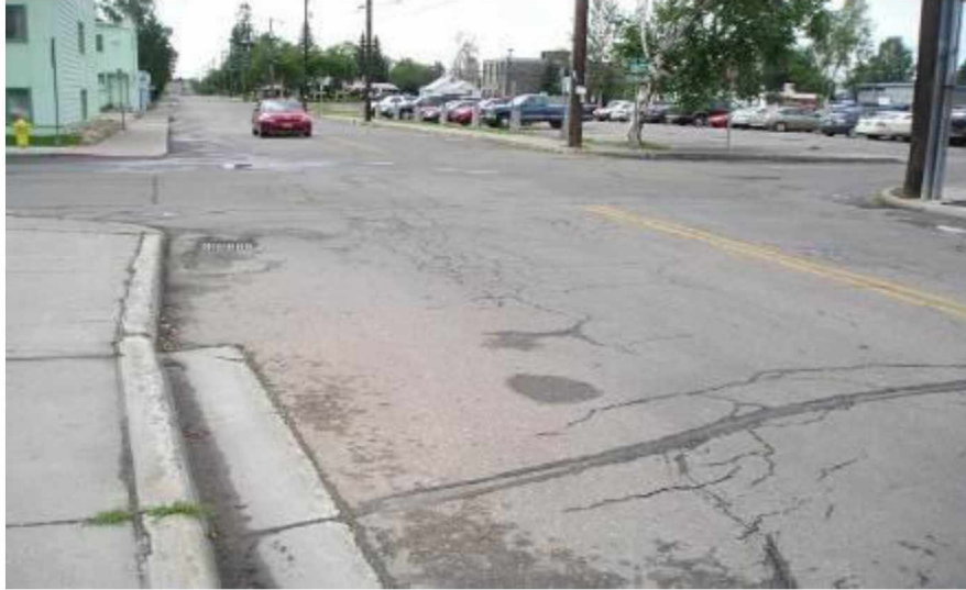
Figure 3.6: Lacey Street, Fairbanks, crack seal, thermal cracking, and alligator cracking, 2011.
