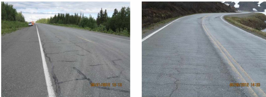
Figure 3.14: Examples of lesser thermal cracks.
