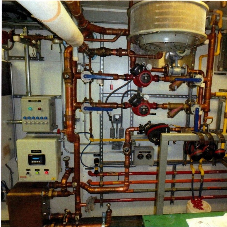
Figure 5. Heat Recovery System Savoonga, Alaska.
