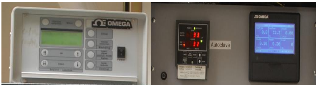
Figure 31: Omega Gas Flow-Rate and Temperature Control System
