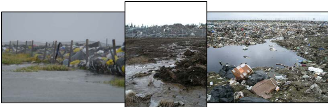
Figure I-3: Surface water at landfill site (left) standing water; and seasonal flooding event at the landfill site (right).
