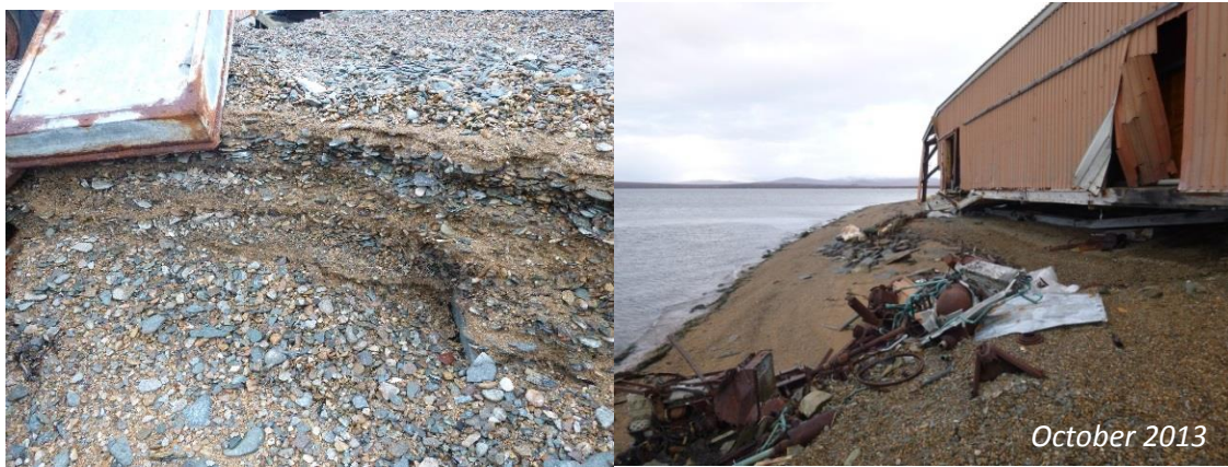
Figure 2.10— Intertidal scarp formed during Oct. 2013 storm near Profile 8, on lagoon side of spit.
