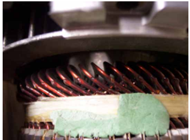
Photo H: View of the protective frame around the electric motor.
