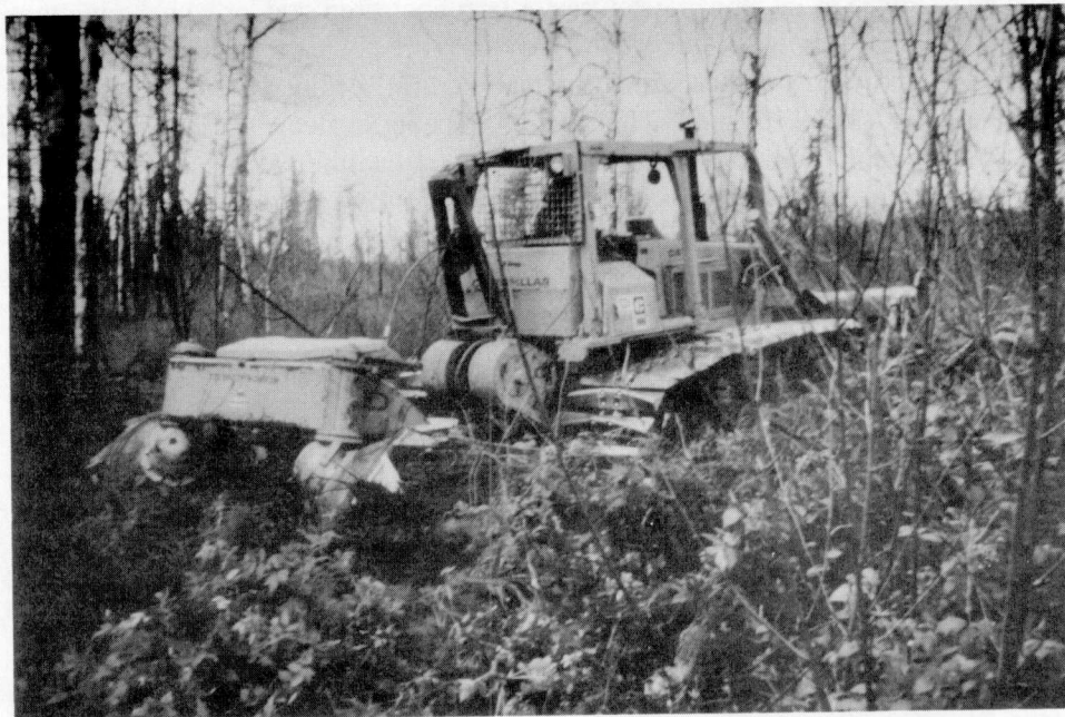
Figure 3. Photo showing the TTS-35 being towed behind the D-6 Caterpillar crawler used by Contractor #2.
