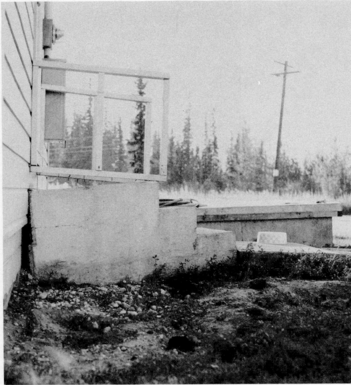
The back steps of the Soil Conservation Service building in Fairbanks are settling due to permafrost melting over a 3-year period. ( Soil Conservation Service photo )
