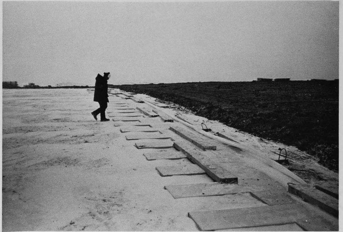
Figure 2. Tunalik airfield under construction in March 1978, showing single layer of 2 inches of insulation and plastic membrane over frozen subgrade.
