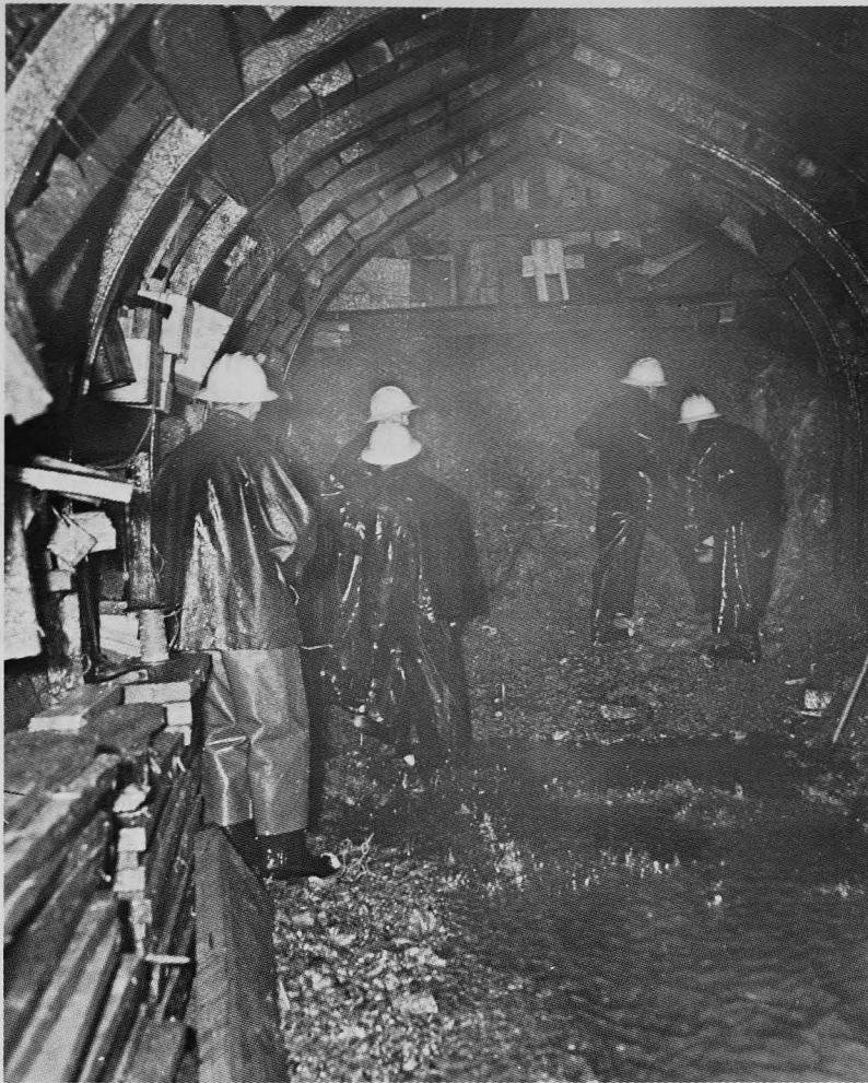
A final check being made in the wet weather under Goat Mountain before blasting on the north heading of Eklutna tunnel.
