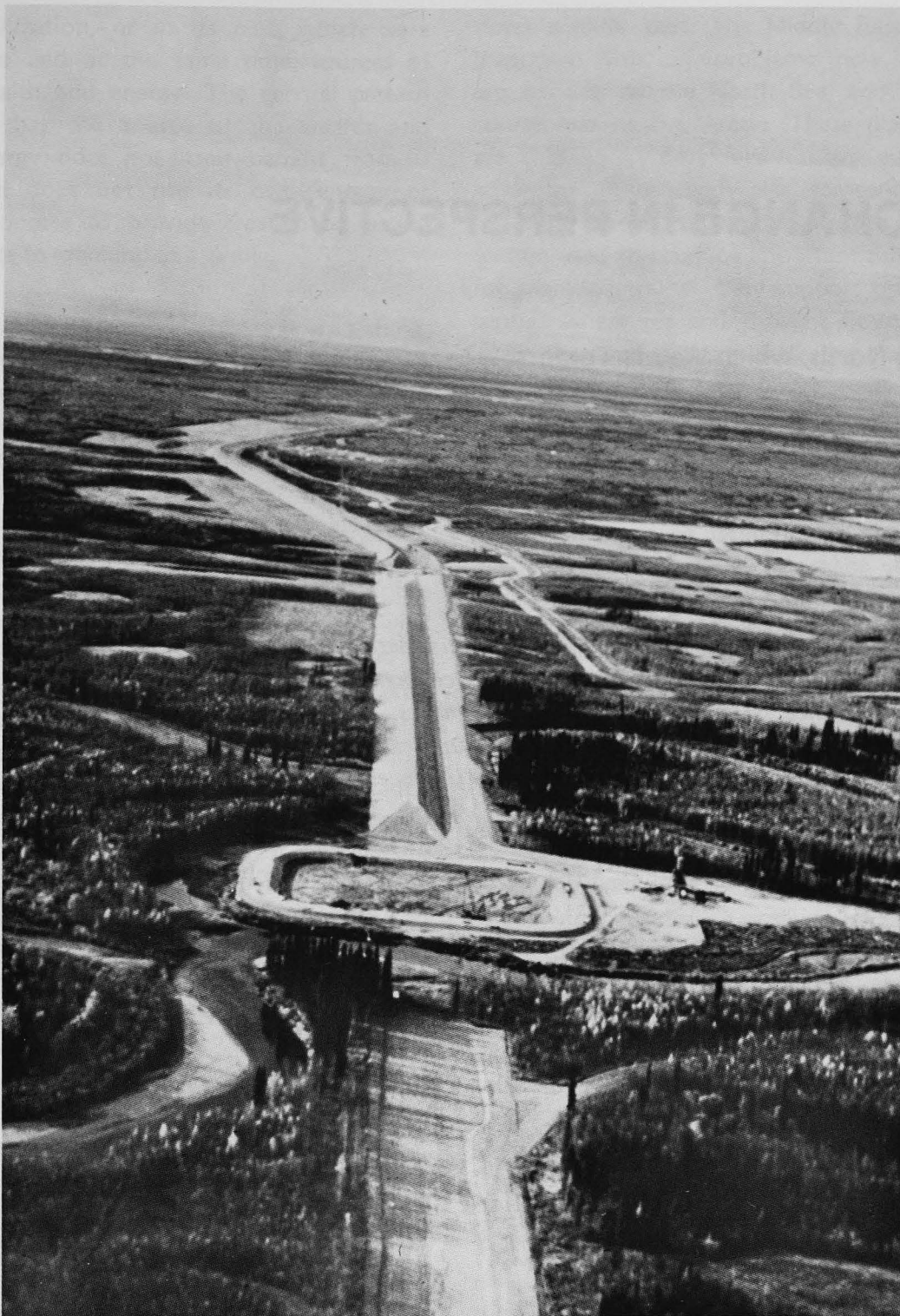
Aerial view looking southeast to the Tanana flats along the Moose Creek dam alignment. Earth coffer dam in foreground surrounds the control works site.
