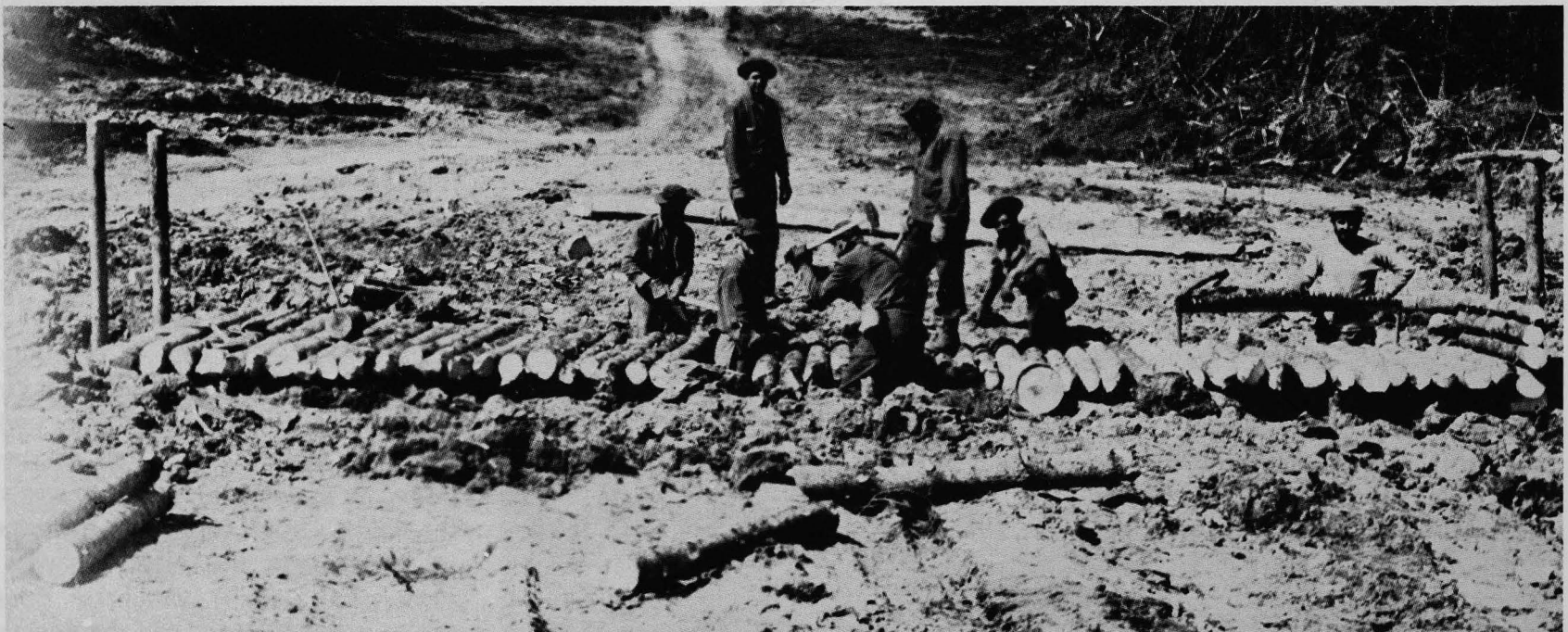
Early culverts were rectangular tunnels built with green timber cut and trimmed nearby. They were replaced later with planks or metal sections.
