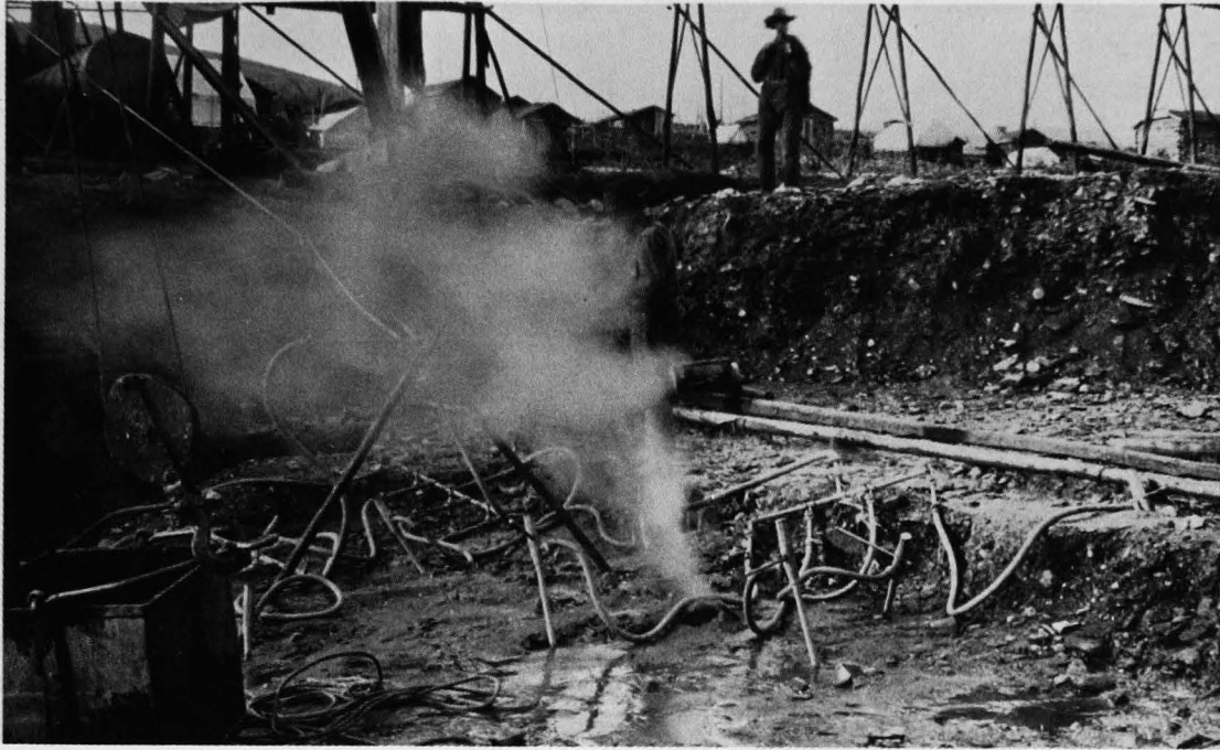
Steam pipes, heated by a wood-fired boiler, are driven into frozen ground to thaw it for digging. (Courtesy of Charles Bunnell Collection, Archives, University of Alaska, Fairbanks.)
