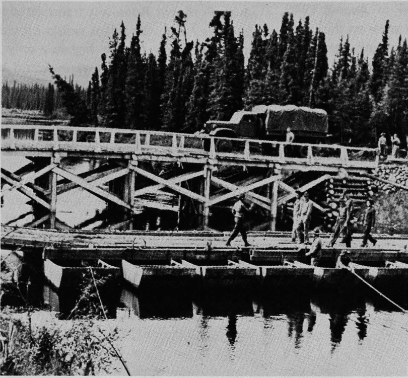
Pontoon bridge over Little Liard River allowed traffic to move forward while the semi-permanent structure was being built.
