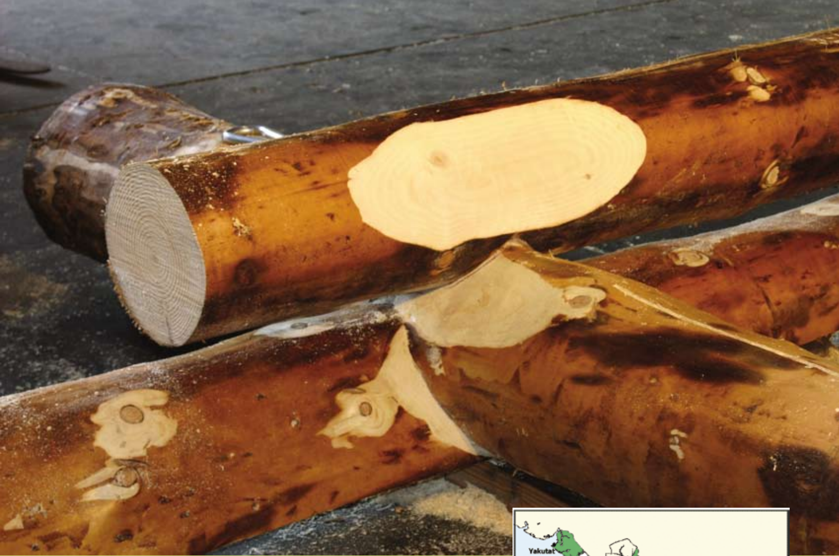
Above: notched logs in the preassembly stage at the hangar on the Sitka campus.
