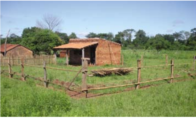
The bamboo fence in progress. Stacked slats are drying in the yard. —PHOTO BY MATTHEW HELT
