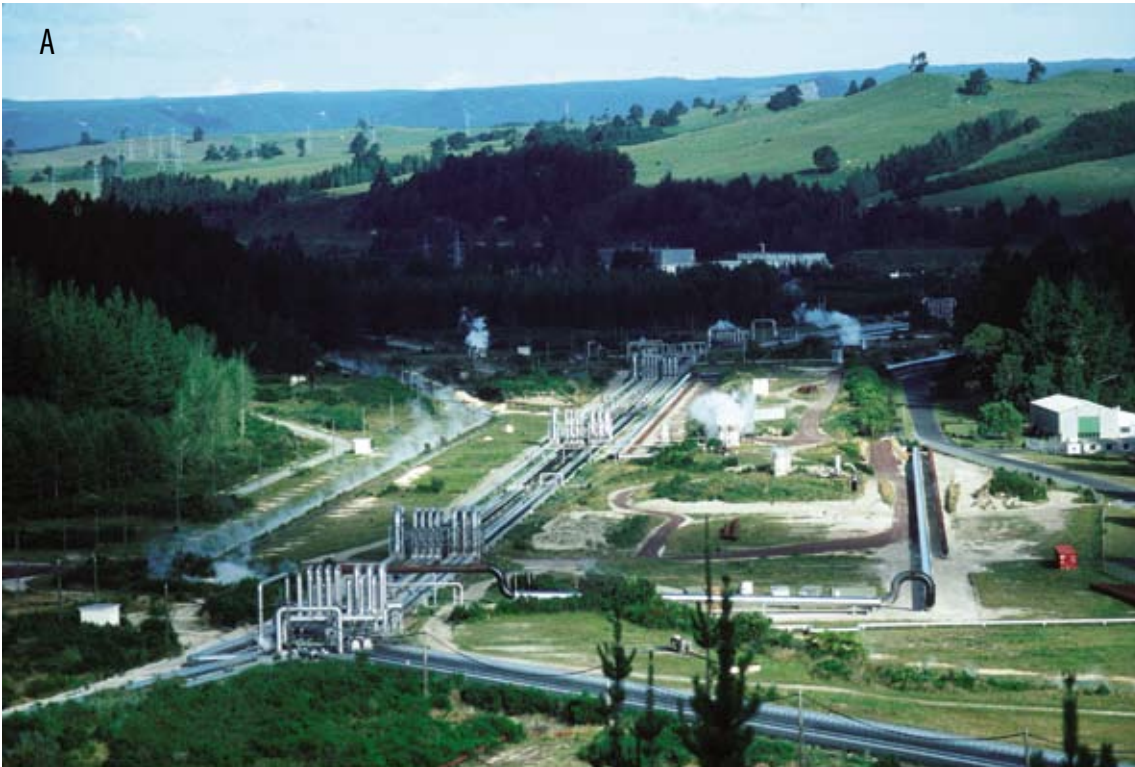
Figure 2. New Zealand's Wairakei Geothermal Power Station project. (A) overview of the geothermal well field and piping, and (B) typical geothermal well infrastructure. —PHOTOS BY KEN BARRICK
