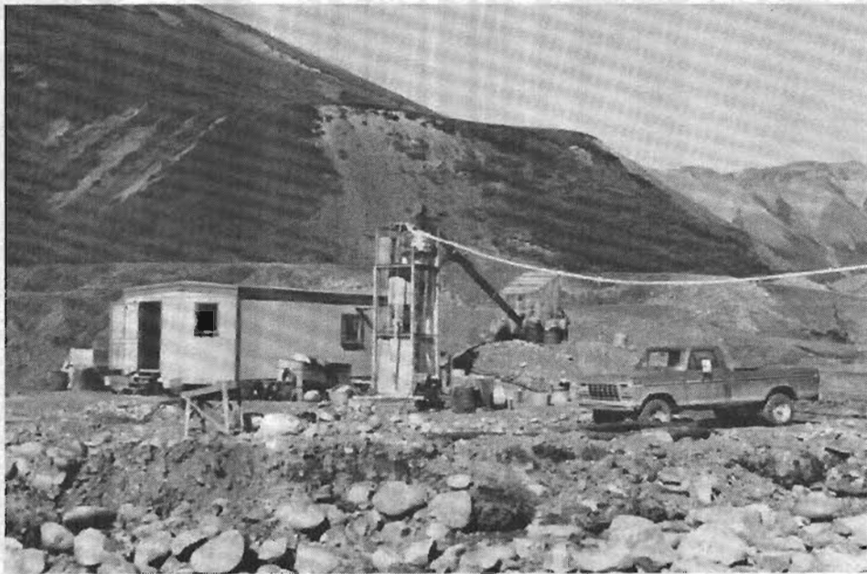
Fig. 17: The clean-up house where gold is recovered from the black sands. The truck brings the black sands to the screw feeder where it is elevated to a 36" three-deck Sweco screen. The minus 24 mesh goes directly to the Deister Table. The plus 24 mesh, minus 14 mesh goes to the pan-o-matic, and the plus 14 minus 1/4" mesh goes to the Denver Panner. The plus 1/4" is panned and inspected by hand.
