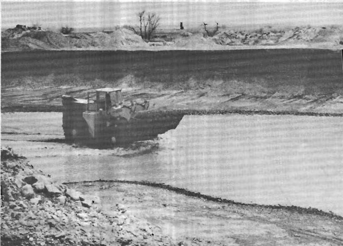
The 15' bank is mined with a front-end loader to the water table. Deposit is about 50 yds from the Snake River, near Grandview, Idaho.
