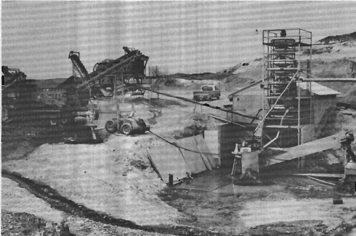
The -3/8" w-shing plant under-size flows down a launder to gravity feed 2 DSM screens, to screen out the +1.5 mm (10 mesh) fraction prior to feeding the cone.
