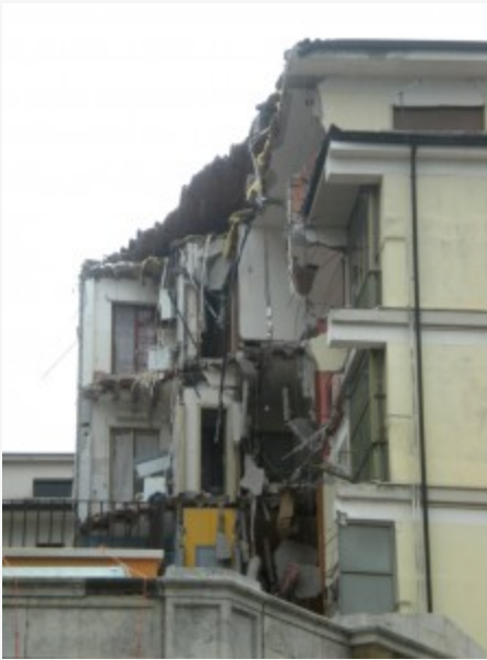
Fig. 12: Collapsed student dormitory (Casa dello Studente), L'Aquila city.
