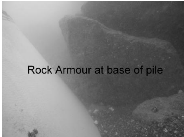
Figure 3.34 – Photographic record of sand and gravel exposure at the monopile wall in Arklow Bank [13].
