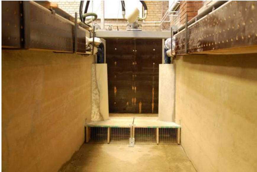
Figure 4.3 – Front view of the pump outlet box plus current distribution box and metal panels (“throat”) to isolate the pipe outlets from the flow.
