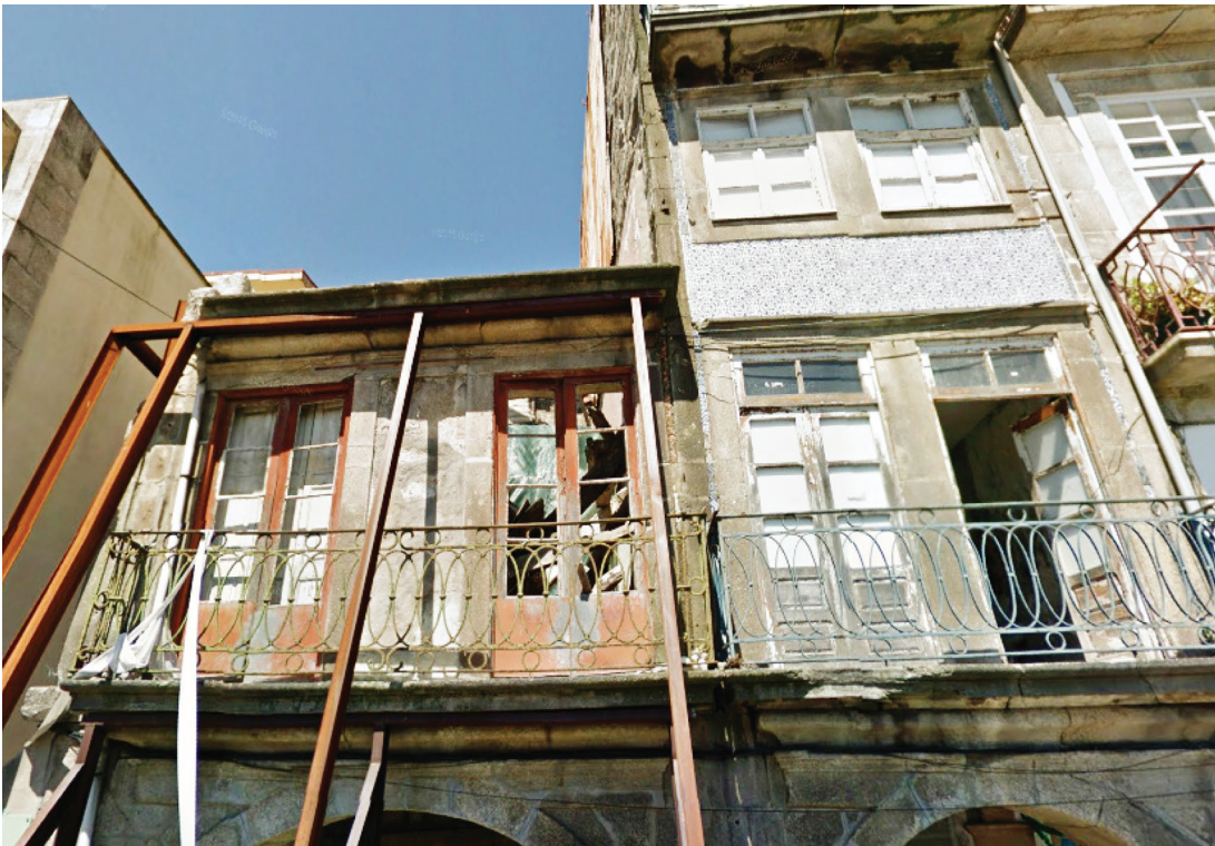
Figure 2 / Degradation of houses in Miragaia. Photo courtesy of Olga Glumac.
