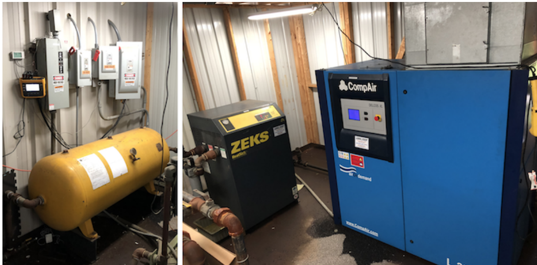
Fig. 2.3. 50 HP Air Compressor System. From Left to Right: Air Receiver, Air Dryer and Air Compressor.
