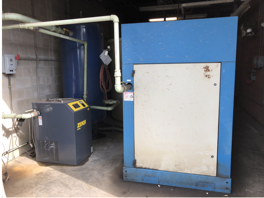
Fig. 2.4. 100 HP Air Compressor System. From Left to Right: Air Dryer, Air Receiver and Air Compressor.
