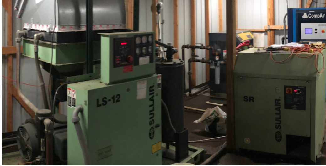
Fig. 3.8. 50 HP backup air compressor.
