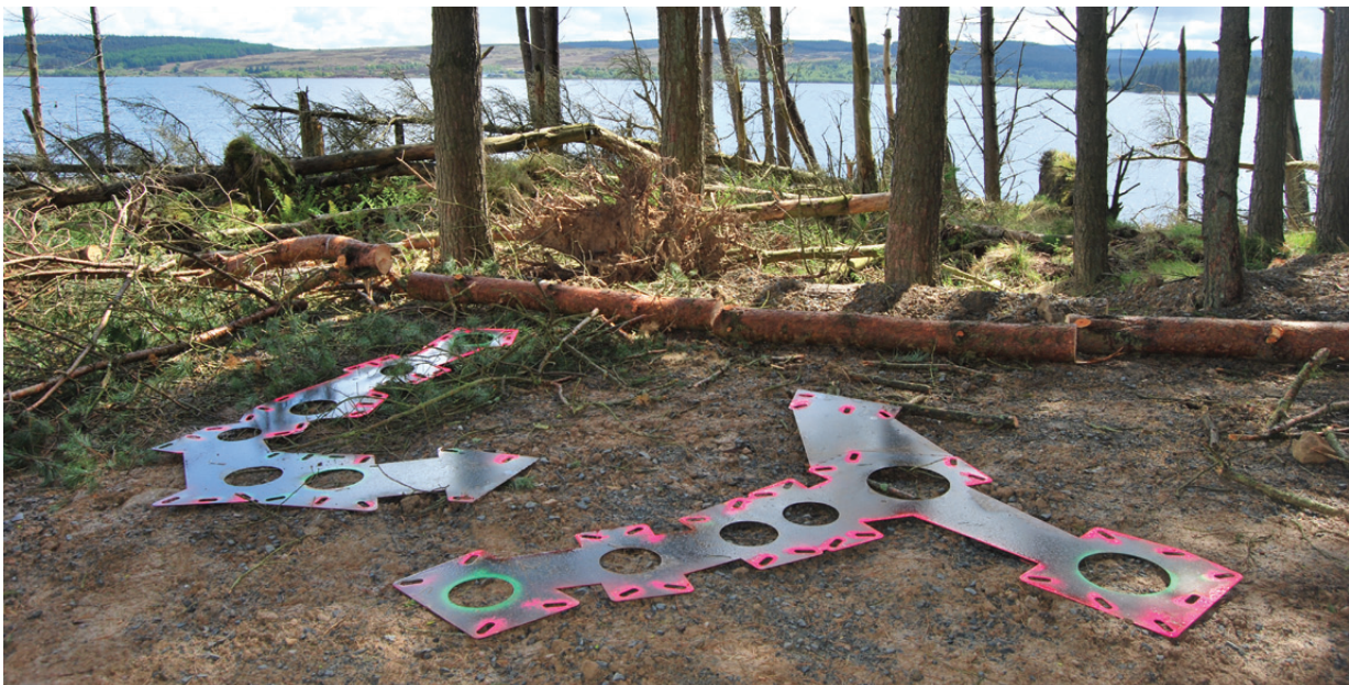
Fig 5.3.18 Manufacturing Protoarchitecture 3: Setting out jigs on site prior to commencement of final assembly of the 55/02 shelter. Such physical tools are entirely derived from the digital file that generates the architectural assembly, and thus act as ‘difference’ verifiers. xxix
