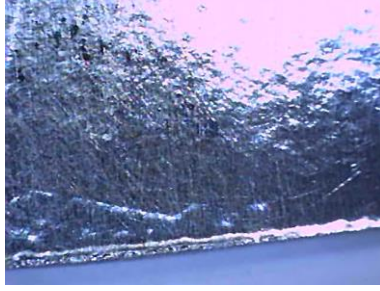
Fig. 4. Porosity and Crack formation of the sample.
